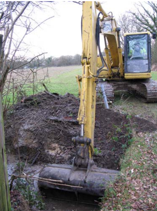
The digger loaned by the Wildlife Centre to clear out the old rotten sleepers from the stream. It came with driver so we did not get a go!
